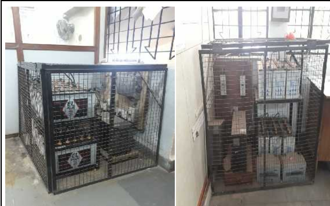
UPS installed for Branch & ATM are well protected & are not accessible for layman. Provision should be made for hydrogen exhaust using exhaust fans.
