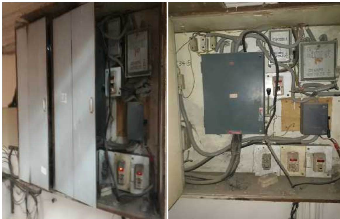
Distribution Boards & Fuse units are installed on wooden board which may catch fire during fault. It is recommended to use metal DB in place of existing wooden board.
